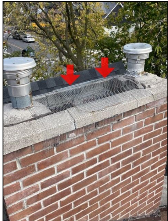
Rain caps missing
