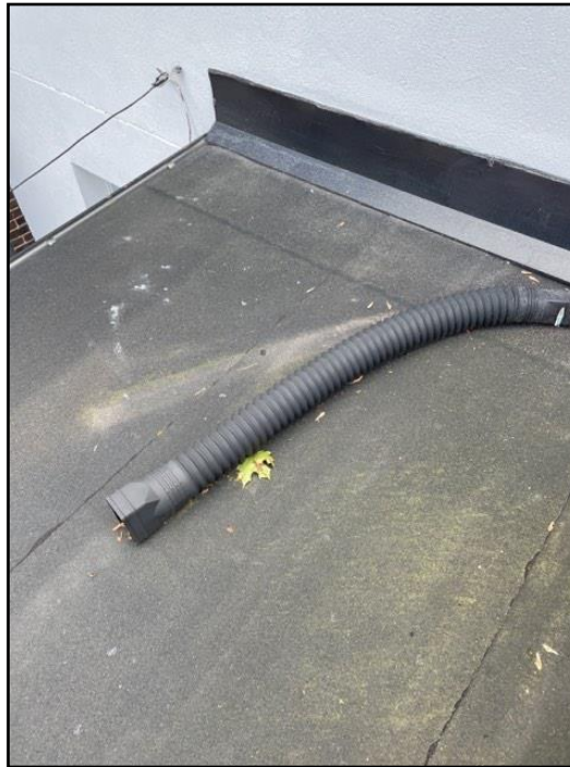
Discharge onto roofs
