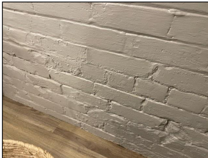
water damaged brick denotes previous leakage
