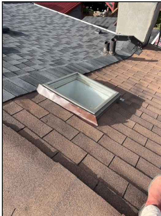
Skylight(s) - vulnerable area for leaks
