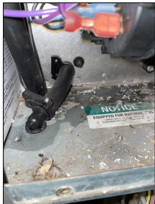
water (condensate) in cabinet
